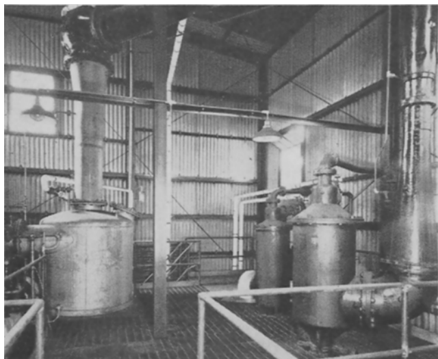
FIG. 5. Vapor scrubber and vacuum system.
